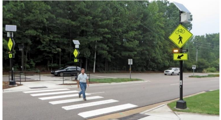
Figure 4. Example RRFB Installation
