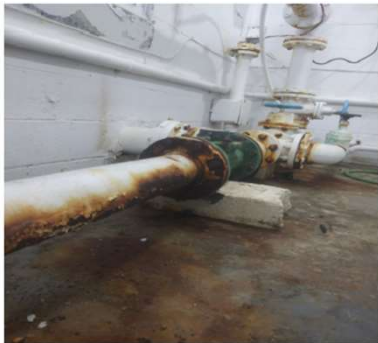
Image 1B: Damaged Supply Line in the North Plant
